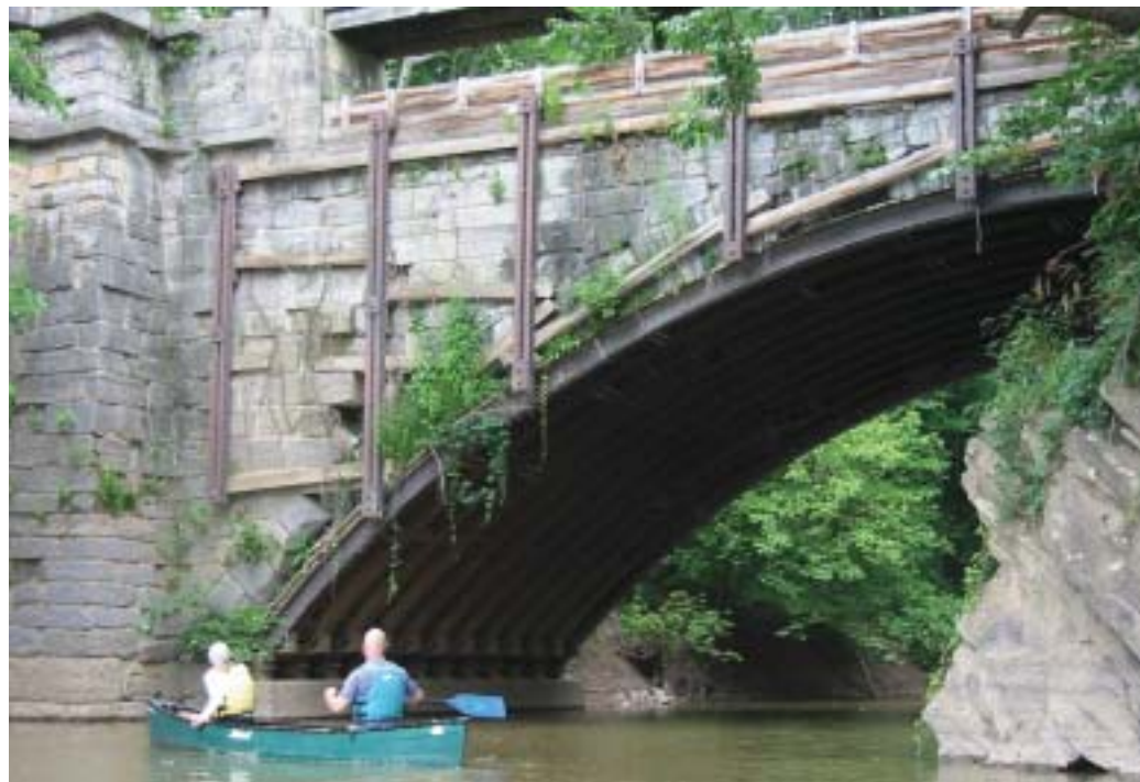
Canoeists paddle under Tonoloway Creek Aqueduct, near Hancock, Md., for a closer look." Photo: J. Dotsen/ICPRB
